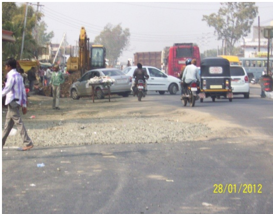
Figure-2 No advance warning signs
