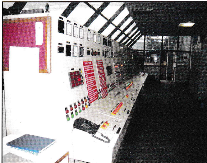
The Control Panel
