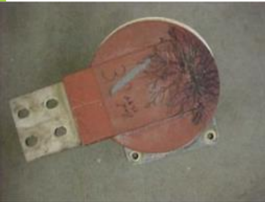
Switchgear Primary Stab Surface Tracking
