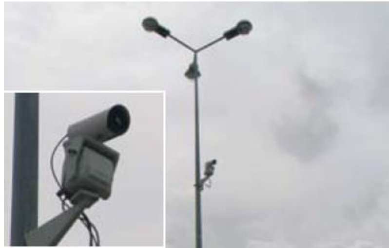
FIGURE 1. Thermal Image Cameras Installed on Port.
